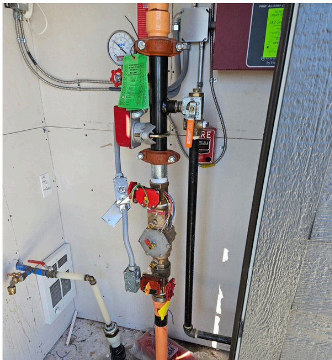
Picture Area 1: Riser Room (Warm Zone)
