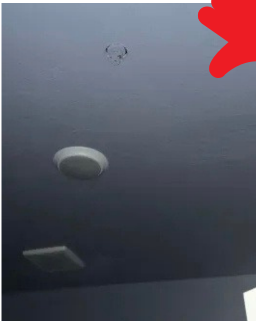
Painted Sprinkler Head (Wrong)
